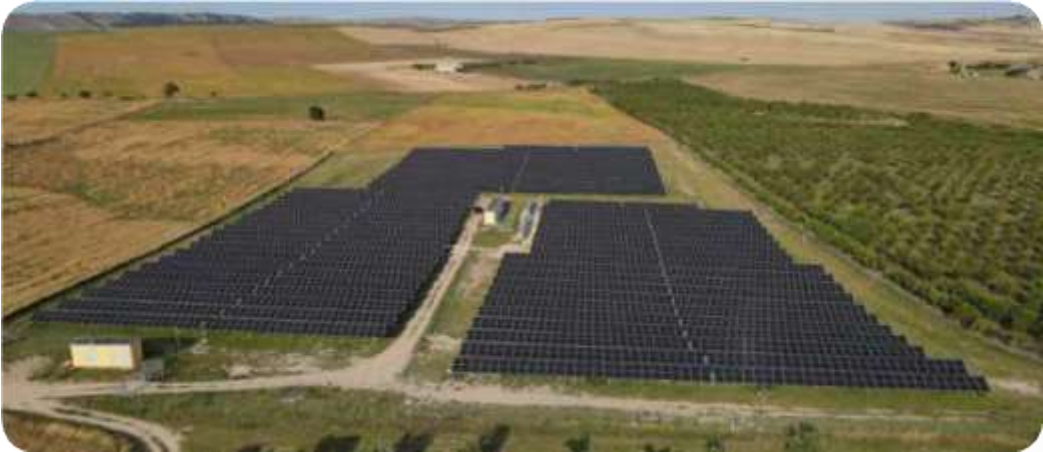
SYSTEMS FOR PHOTOVOLTAIC PARK S1.5 MW plant built with CONTERRA@TRACKER structure
