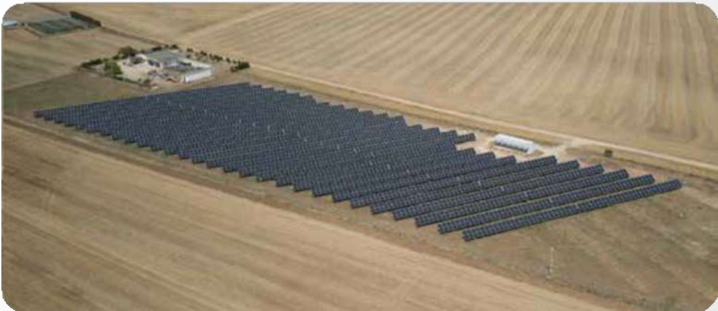
SYSTEMS FOR PHOTOVOLTAIC PARKS 999 kW plant built with CONTERRA@TRACKER structure
