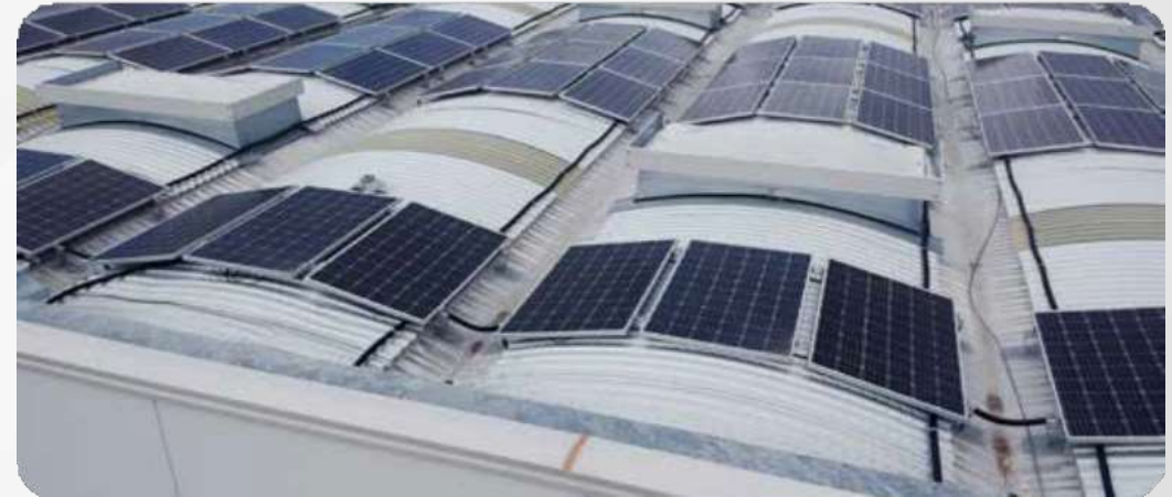
SYSTEMS FOR INDUSTRIAL ROOFS 300 kWp system built with customised supports for domes
