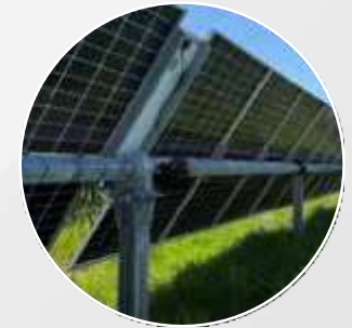
Ground-mounted systems Tracker
