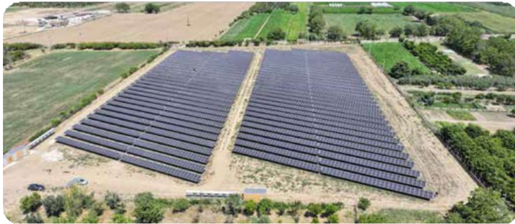
SYSTEMS FOR PHOTOVOLTAIC PARKS 2 MW plant built with CONTERRA@TRACKER structure
