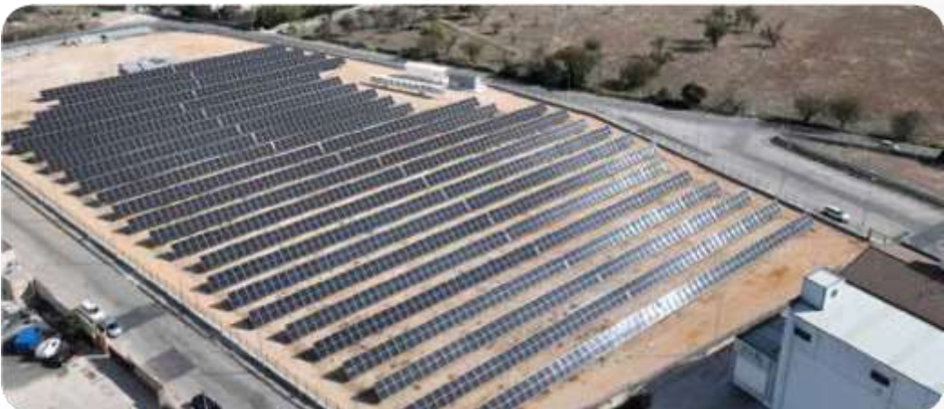
SYSTEMS FOR PHOTOVOLTAIC PARKS 950 kW plant built with CONTERRA@TRACKER structure
